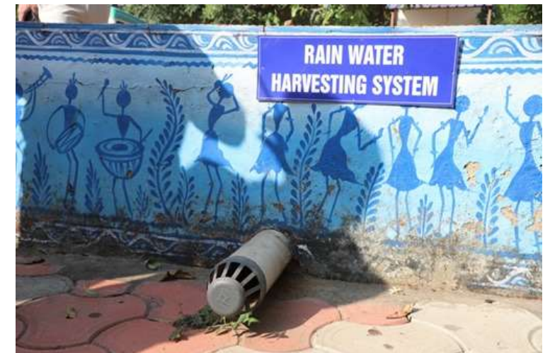
Rainwater Harvesting in UPHC-4, Bhubaneswar, Odisha
